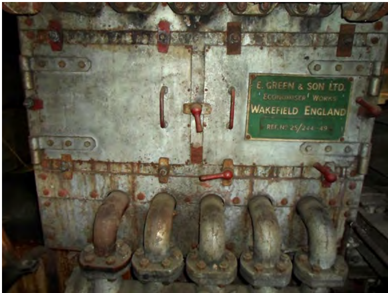
A 1940's 'Green's Economizer' in a boiler house in Launceston, Tasmania. Image courtesy of Wriekhathaar
